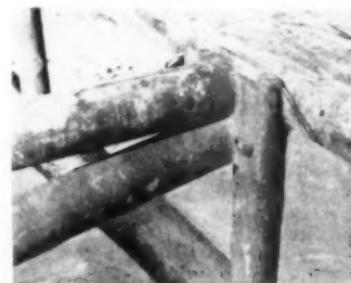
SOLID SUPPORT. —Section bolted to side rail of walk, above, provides a continuous support for drill pipe and casing.
